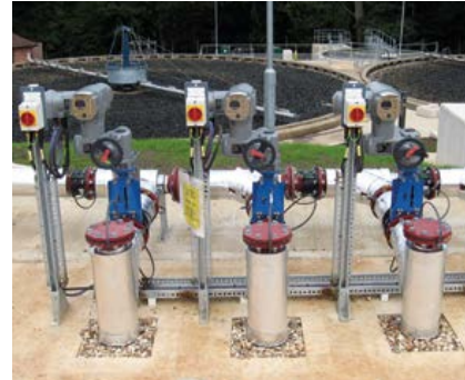
Cabling, containment and isolators for power and profibus driven actuated valves.
