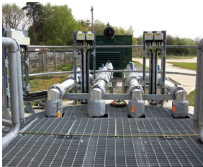
Power, control and instrumentation installed for a new wastewater pumping station and generator.
