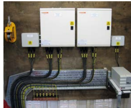
Power distribution, earthing and UPS for actuated valves and forklift charging point within a factory.
