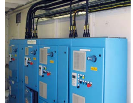
Installation of new MCC, cabling and containment work for a new wastewater pumping station.
