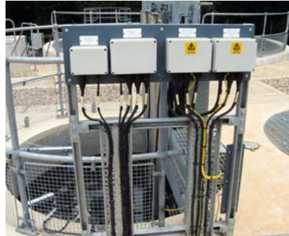
Cabling and containment for installation of instrumentation and motors for a new re-circulation pumping station.
