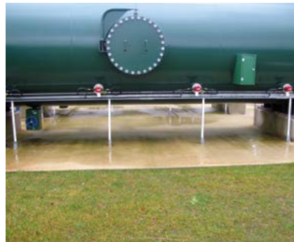
Cabling and containment for power supplies to heaters for a new surge vessel.
