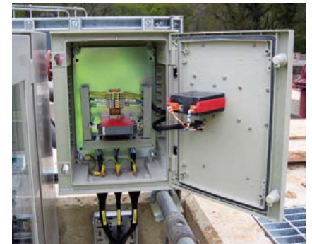
Cabling and cabinet for a Full Flow to Treatment MCERT flowmeter repeater for the EA.
